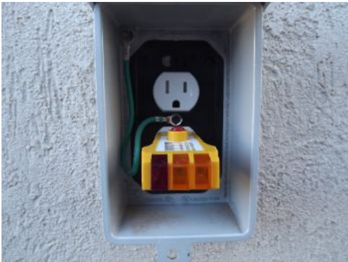
Exterior outlet (by main panel) was not functional, recommend correction by licensed professional
