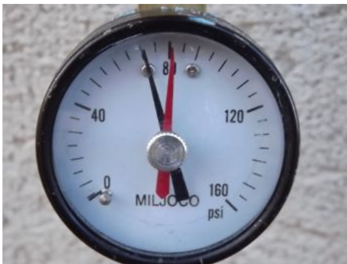
Static Water Pressure Reading: 78 PSI
